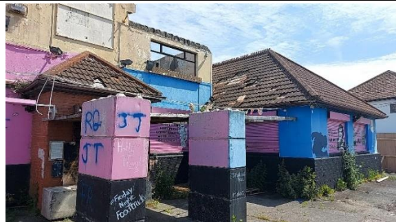
Photograph 4. Existing derelict building and BL3 habitat in the southern section of the Site (17 th June 2025)
