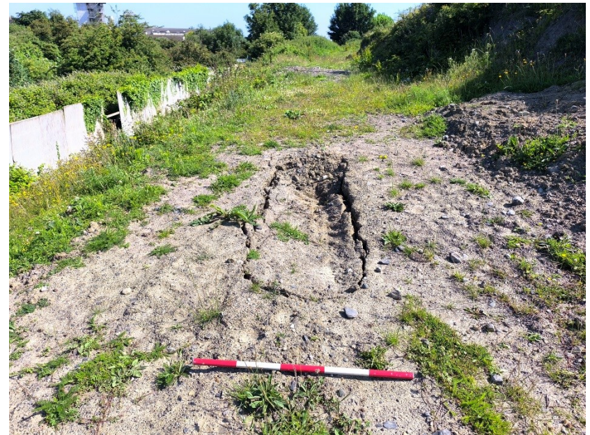
Plate 20: View of damaged ground and uneven site from previous works on site, facing north
