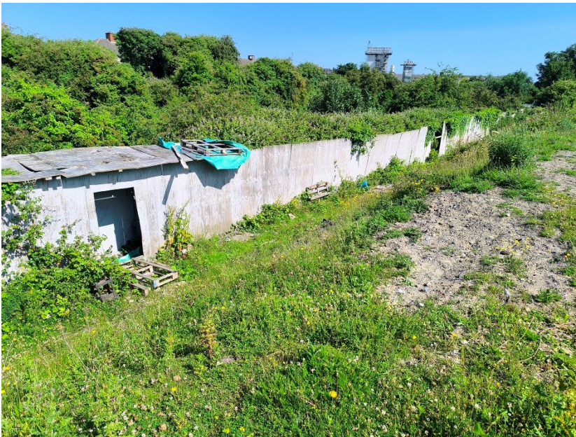
Plate 19: View of broken hoarding along western boundary with railway line, facing northwest
