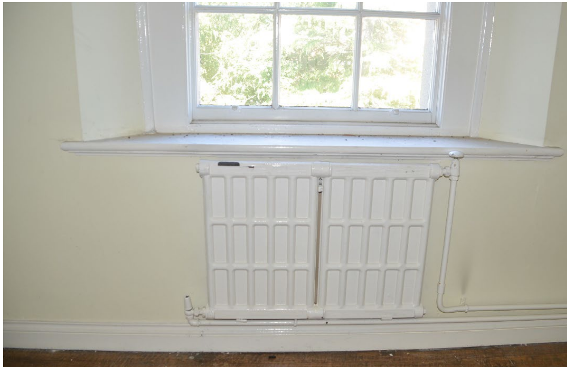
Figure 42: Photo showing a surviving cast-iron radiator within the New Wing. There are several surviving examples of this type of radiator throughout first and second floor levels.
