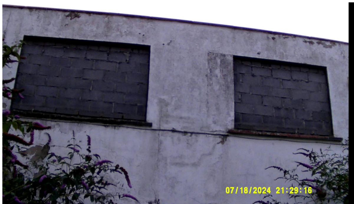
FIGURE 6. PRF 3 – BRICKED UP WINDOWS.
