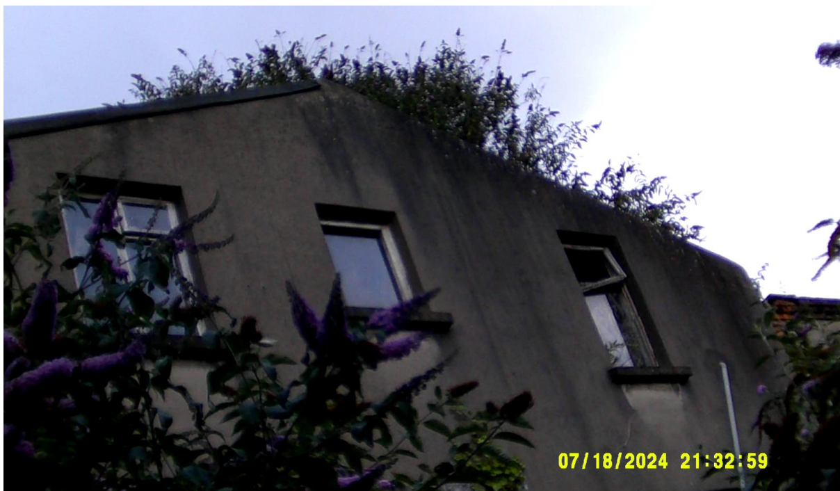
FIGURE 5. PRF 2 – A BROKEN WINDOW.
