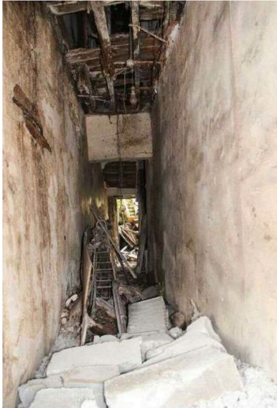
Plate No. 63. General view showing ground floor entry hall to No. 46 Dolphins Barn Street as it appeared in 2017. The dangerously rotted floor joists above show how far this house has deteriorated. This structure is now too dangerous to enter, other than the entry hall. (Photo by Stephen Farrell, 2017)
