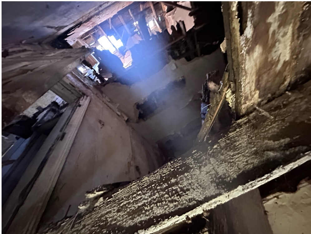
Plate No. 66. General view up from the rear of the first half landing, in No. 46 Dolphins Barn Street as it appeared in 2017. A close study of this photo shows that all of the internal timber floor and the roof structure was replaced during the 20th century, along with all joinery and linings. This structure is now too dangerous to enter, other than the entry hall. (Photo by Stephen Farrell, 2017)
