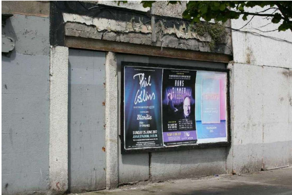
Plate No. 52. Detail view showing the poor quality shopfront to No. 44 Dolphins Barn Street as it appeared in 2017. Door at left opened into the entry hall, and another door served the shopfront. Note the steel RSJ that supports the upper floors. (Photo by Stephen Farrell, 2017)
