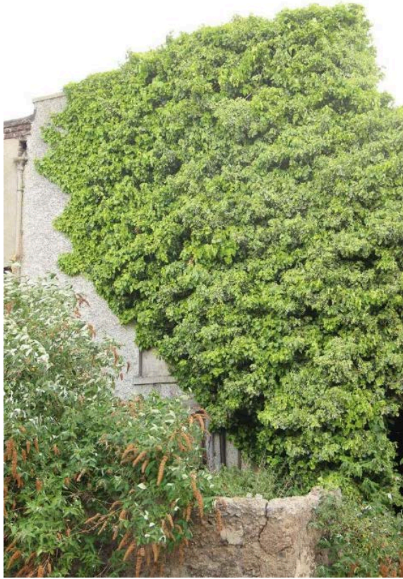
Plate No. 27. General view showing the rear elevation to No. 44 Dolphins Barn Street in 2017. The thick growth of ivy has obscured most of the surface of the rear, however the sand and cement dashed render, and granite coping slabs on the parapet are visible. (Photo by Stephen Farrell, 2017)
