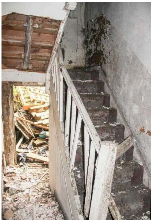
Plate No. 64. Detail view showing the poor quality replacement stair to No. 46 Dolphins Barn Street as it appeared in 2017. (Photo by Stephen Farrell, 2017)
