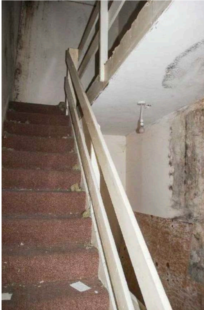
Plate No. 54. Detail view showing the poor quality 20th century stair in No. 45 Dolphins Barn Street as it appeared in 2017. There is no trace of the 18th century stair. (Photo by Stephen Farrell, 2017)
