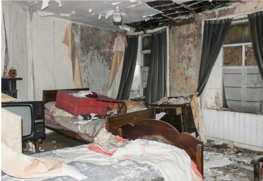
Plate No. 46. Detail view showing the second floor front bedroom in No. 44 Dolphins Barn Street as it appeared in 2017. The corner chimney breast is at the left, with a good quality slate fire surround. That area has been heavily damaged by damp rot and dry rot fungus. (Photo by Stephen Farrell, 2017)
