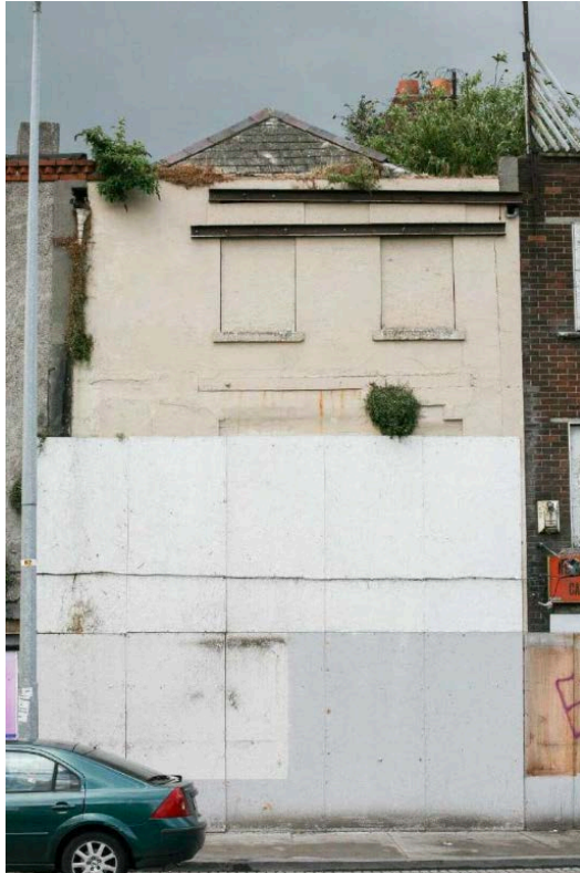
Plate No. 60. General view showing the front elevation to No. 46 Dolphins Barn Street with steel braces fixed to the front parapet. Note the low pitched slated roof and the odd position of the windows in the elevation. It is likely this house was built as a group with Nos. 44 and 45 by the same builder around 1725-1750 (Photo by Stephen Farrell, 2017)
