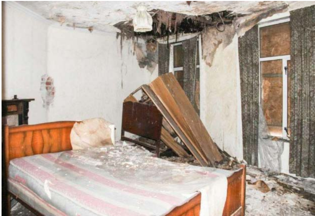
Plate No. 37. General view showing the first floor front room in No. 44 Dolphins Barn Street, in 2017. Note the late 19th or early 20th century fireplace in the angled chimney breast at left. Also note the extensive damage caused by unchecked roof leaks in the front roof. (Photo by Stephen Farrell, 2017)
