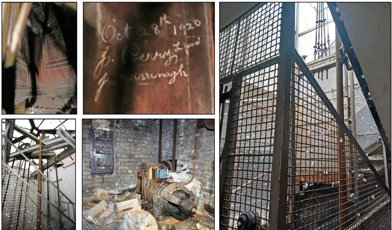
Fig 2.8 Passenger lift in Abbey Buildings. Clockwise from top left : Cage interior (obstructed by the landing door); 1920 inscription on cage panel; Maker’s name on counterweight ( photo courtesy Molloy Associates ); Motor in basement; Hoist rope pulley in lightwell at top of lift shaft.
