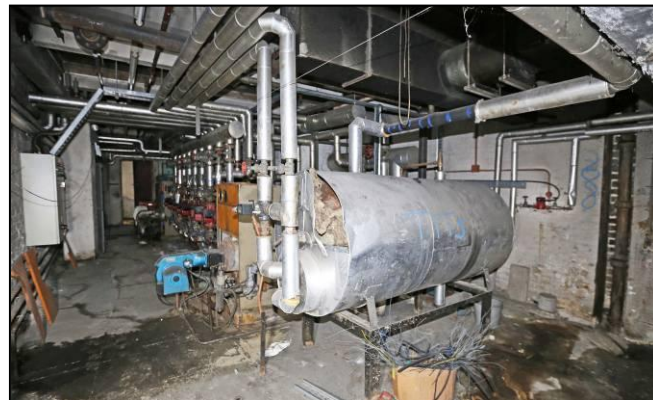
Left: Ideal Standard 'Viceroy' boiler towards south end of room.
