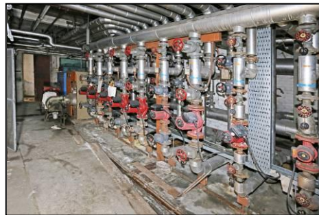
Left: Buderus boiler (left) and Ideal Standard 'Viceroy' boiler at north end of room.
