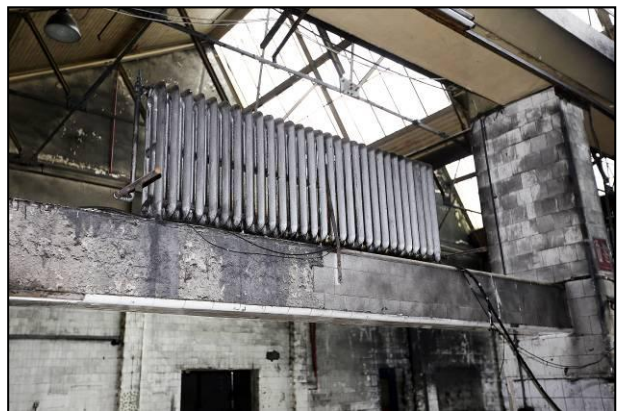
Radiator mounted on rfc beam between bays.
