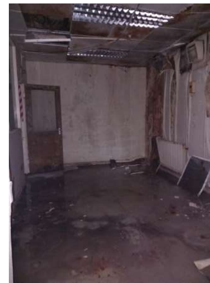
Plate 143: Rear ground floor of 87-90 Middle Abbey Street. Area is in poor condition due to water ingress.
