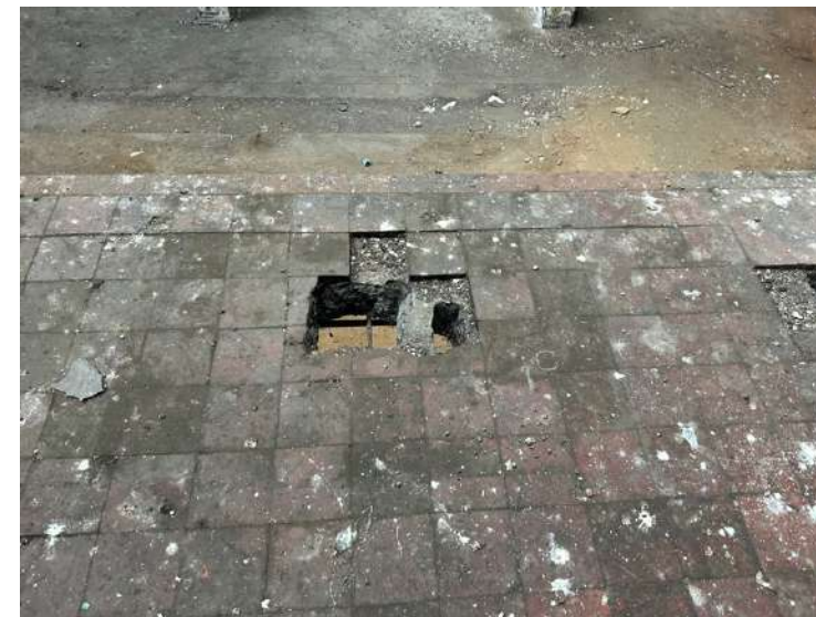
Plate 208: Detail of balcony overlooking machine room floor. Quarry tiles on concrete balcony overlooking Printing Hall. A number of balconies have been partially demolished.
