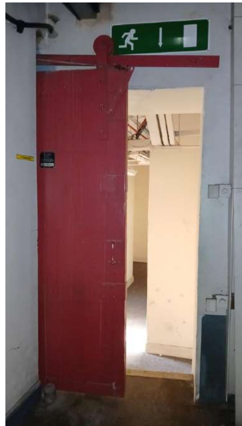
Plate 12 Steel fire doors separate the connections between Independent House and Emerald Chambers.
