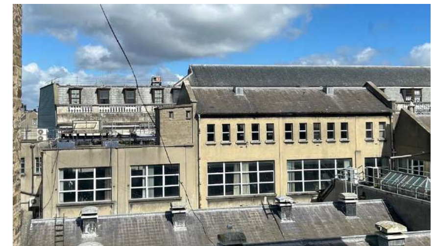
Plate 24: Zone 4b, Rear elevation of the former distribution centre and offices for Independent Newspaper group, fronting onto Prince's Street North. Replacement uPVC windows throughout.
