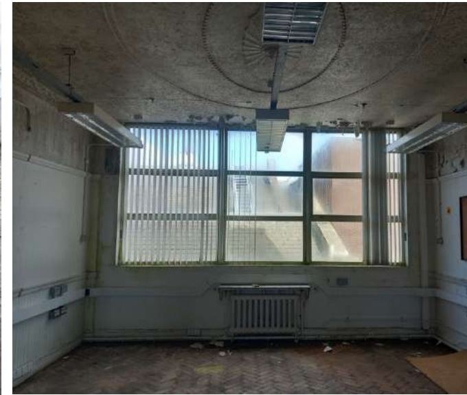
Plate 77: View facing north in former boardroom. Replacement uPVC windows and exposed contemporary services throughout. Moulded timber skirting, dado and picture-rail. Neo-classical plasterwork to ceiling in regency style. Original parquet floor, damaged by water ingress.
