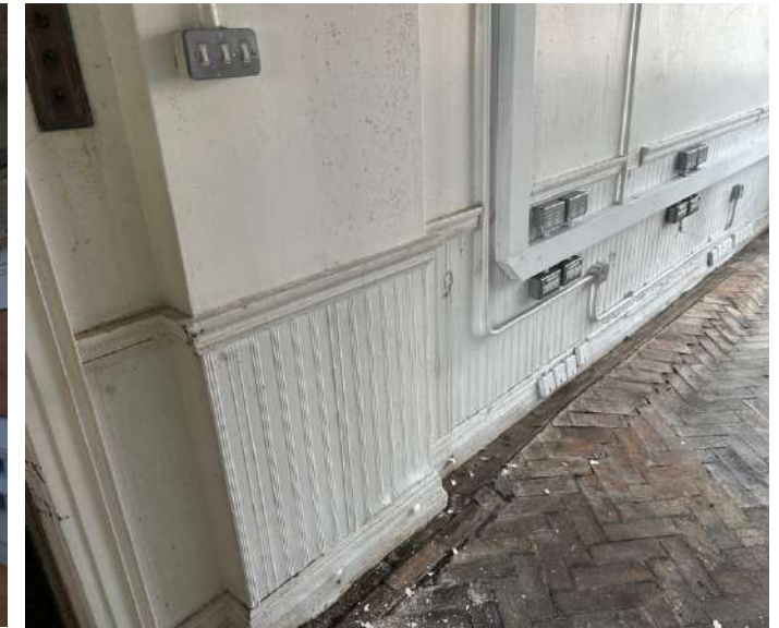
Plate 78: Moulded timber skirting, dado and picture-rail. Neo-classical plasterwork to ceiling in regency style. Original parquet floor, damaged by water ingress.
