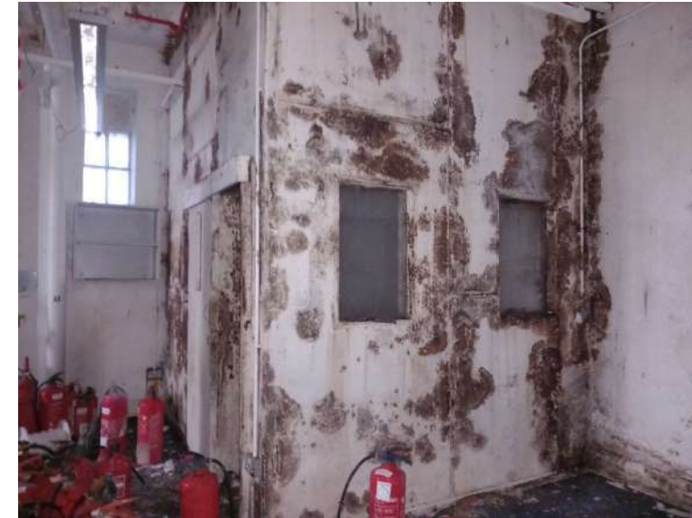
Plate 137: Contemporary partition forming internal room. Steel window to William's Lane. The structure has been impacted by water ingress in this area and the condition of embedded steel in concrete frame to be examined by engineer.
