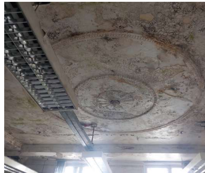
Plate 80: Neo-classical plasterwork to ceiling in regency style, damaged by water ingress from roof.
