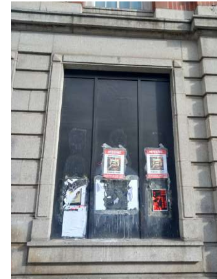
Plate 116: Ground floor window, boarded up windows, opening framed with cut granite architrave with diamond faced blocks.
