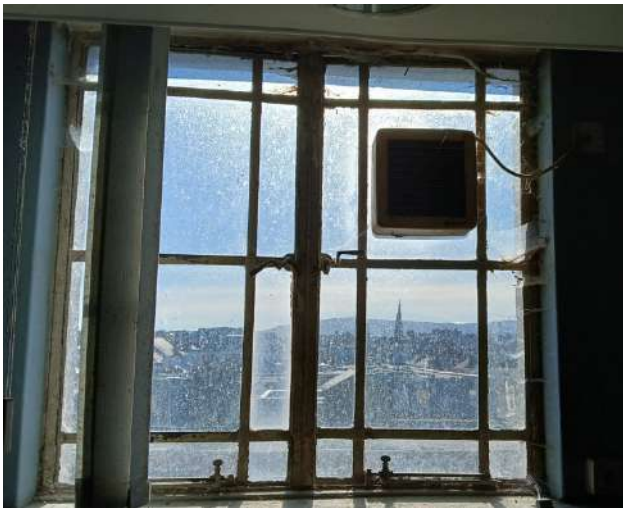
Plate 98: Only one original window remains at level 4, all others have been replaced,
