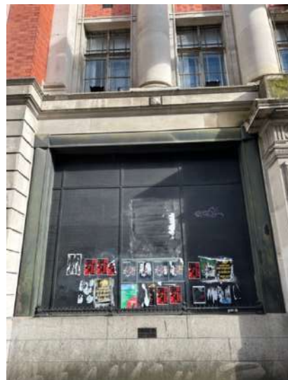
Plate 7: Bronze window surround with diamond shaped blocks.
