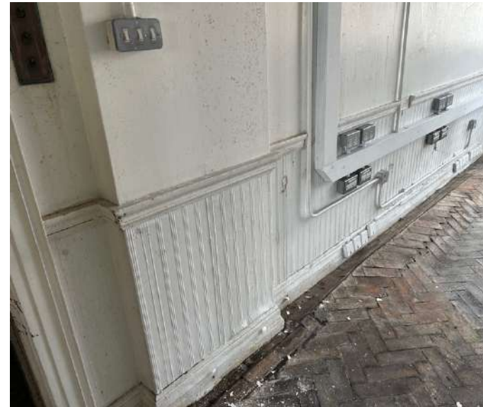
Plate 76: Moulded timber skirting, dado and picture-rail. Neo-classical plasterwork to ceiling in regency style. Original parquet floor, damaged by water ingress.
