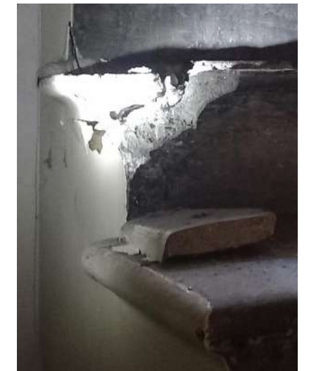
Plate 7 Impact damage at the entrance hall reveals the composition of the stairs to be concrete with a polished composite layer applied.
