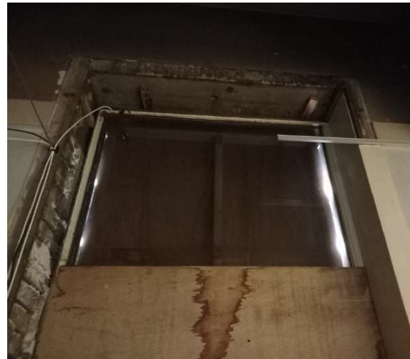
Plate 43: Window frames and architraves missing from entrance lobby.
