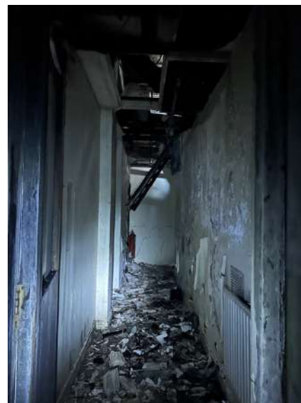
Plate 141: The derelict condition of the rooflights has resulted in extensive damage to the building fabric.
