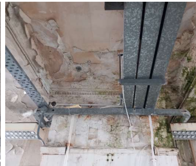
Plate 81: Neo-classical plasterwork to ceiling in regency style, damaged by water ingress from roof. Downstand beams with decorative cornice. Exposed contemporary services fixed through ceiling fabric.
