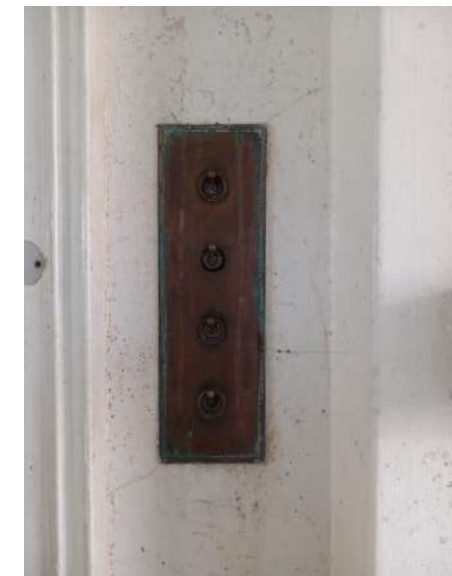
Plate 82: Bronze switch plate with toggle switches in former boardroom.
