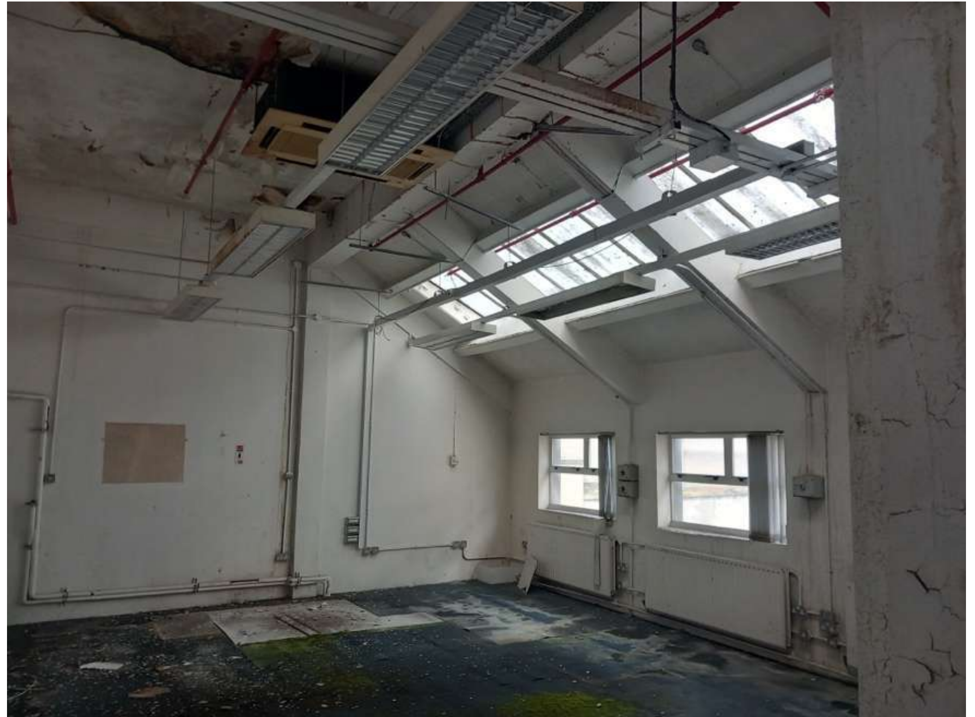
Plate 268: Zone 4, second floor annex. North facing rooflight and pitched profile exposed internally. Contemporary windows onto Prince's Street North, contemporary services and raised access floor throughout. Damage due to water ingress evident.
