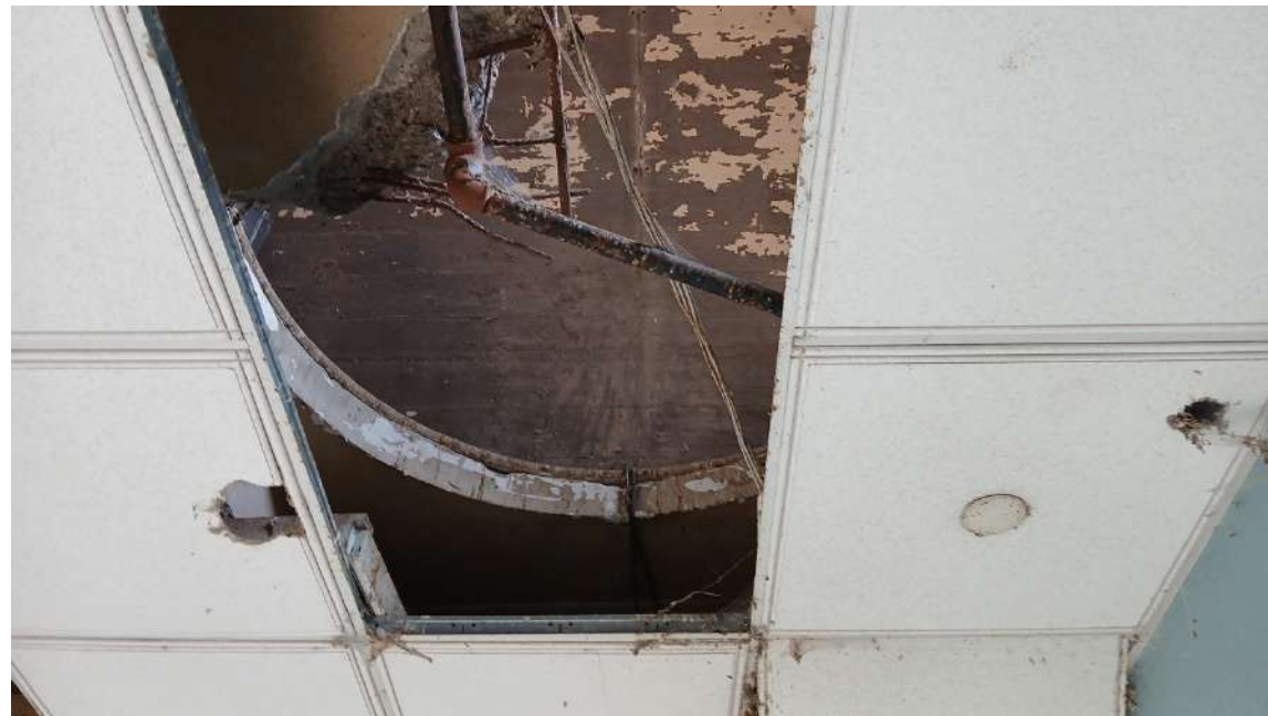
Plate 32: There is no direct roof access to the dome on the east. Historically, access was provided from 4 th floor below, as indicated by the clean circular to the concrete slab, concealed above the contemporary suspended ceiling. Note the partial demolition of roof slab structure, exposing the internal rebar, which has corroded.
