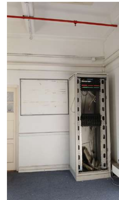
Plate 53: Contemporary services including sprinkler system and heating pipework installed through partition walls.
