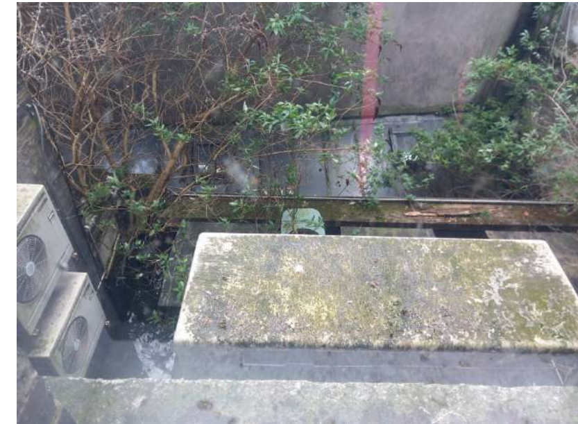
Plate 119: The lightwell is in very poor condition resulting in water ingress impacting the lower-level rooms.
