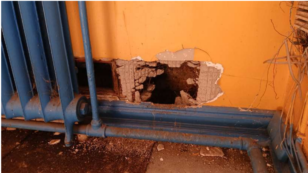
Plate 70: Installation of later services, heating system and pipework, routed indiscriminately through original joinery, partition walls etc. Breach in wall fabric exposing composition of front wall: masonry structure with timbered framed wall lining internally.
