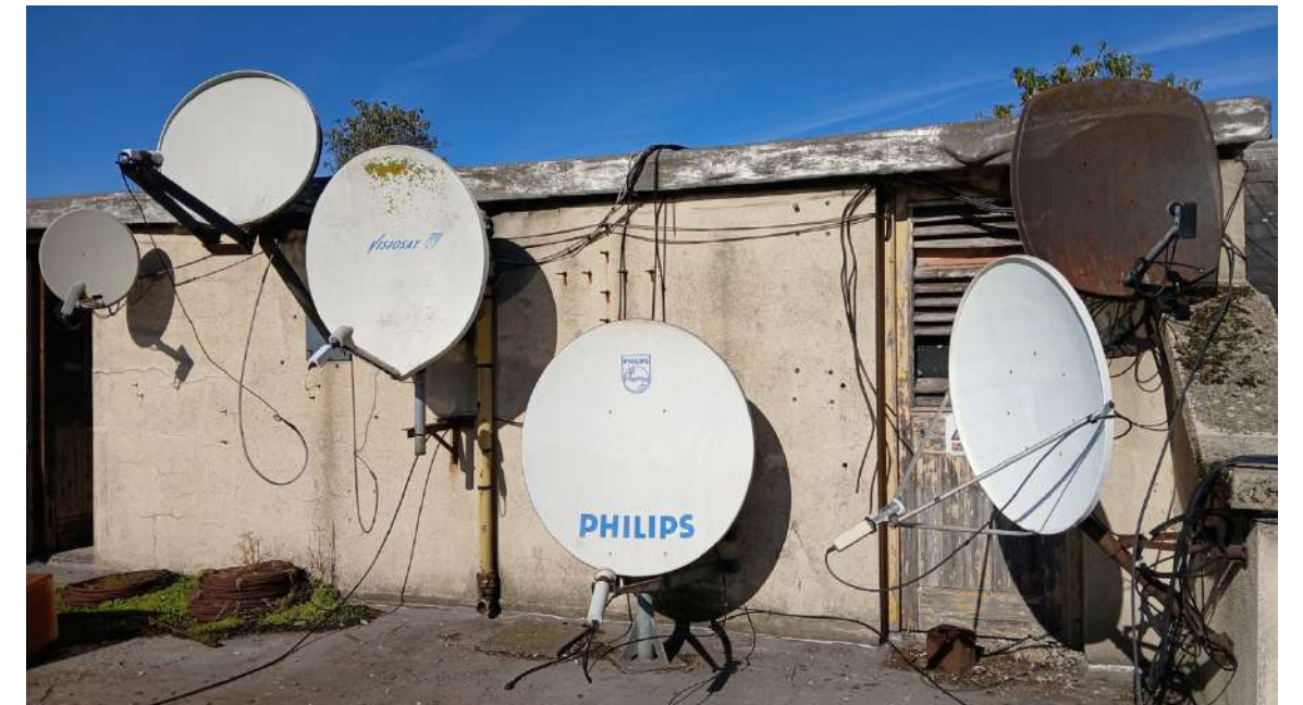
Plate 33: Collection of satellite dishes surface fixed to roof access.
