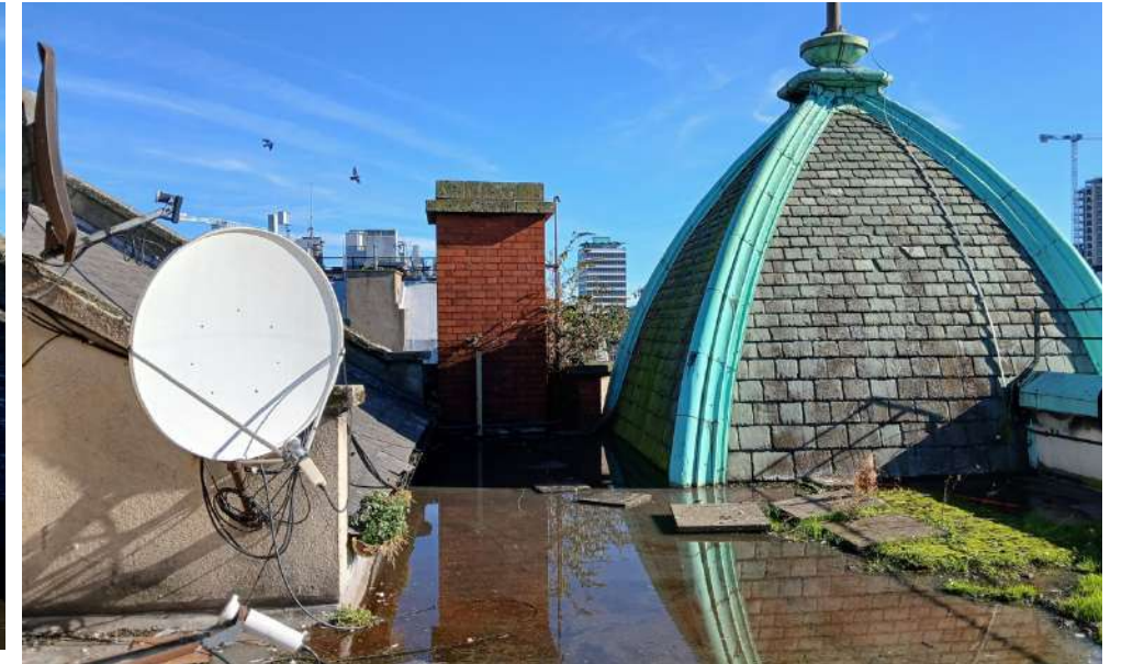
Plate 24: Brick chimneystack on eastern boundary wall. Note the standing water on the central flat roof section, suggesting blocked drainage. The eastern dome is not accessible from the roof level.
