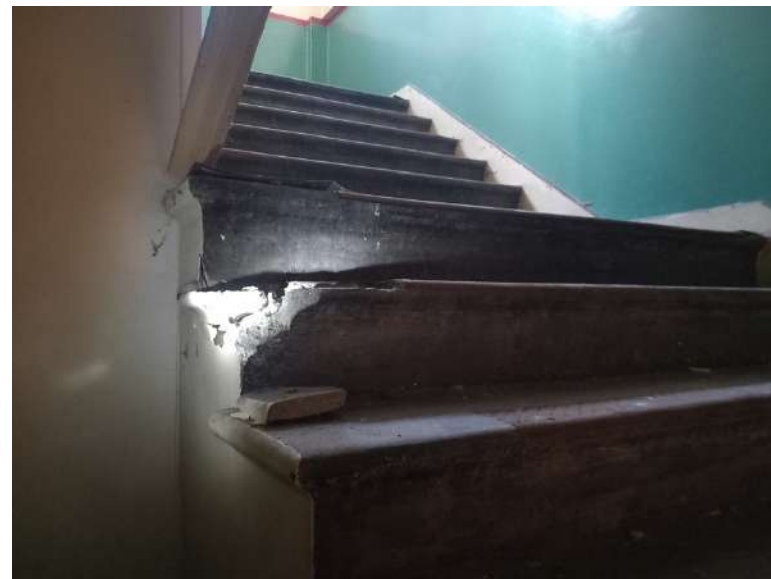
Plate 39: Detail of impact damage to polished concrete stair. Note: handrail and balustrade has been cut and is missing.
