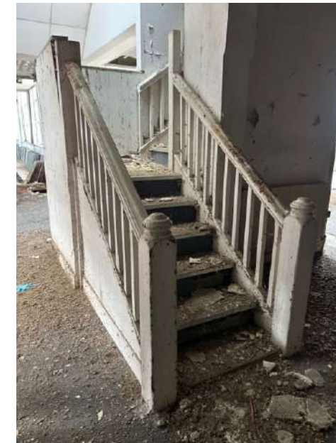
Plate 274: Painted timber stair with square plan newel posts to top floor, possible using salvaged elements.
