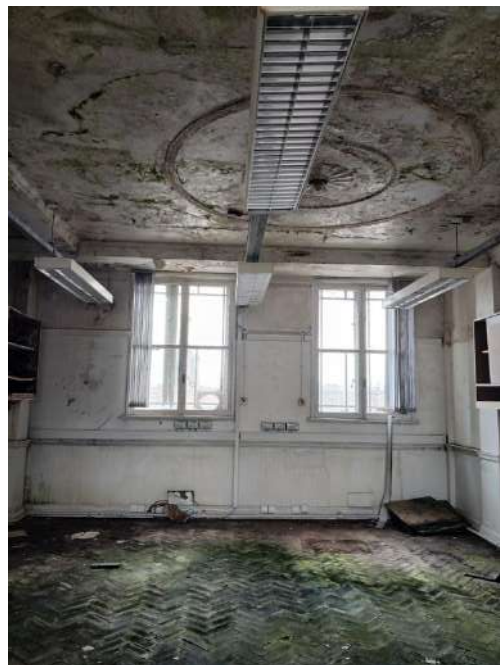
Plate 50 Decorative elements in the former boardroom including the low-relief plaster ceiling and the parquet floor will be repaired where
