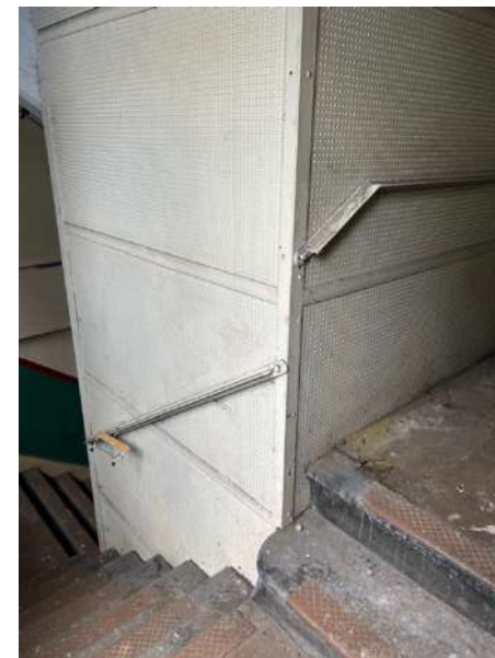
Plate 41: Polished concrete stairs with quarter landings. Handrail missing on upper levels.
