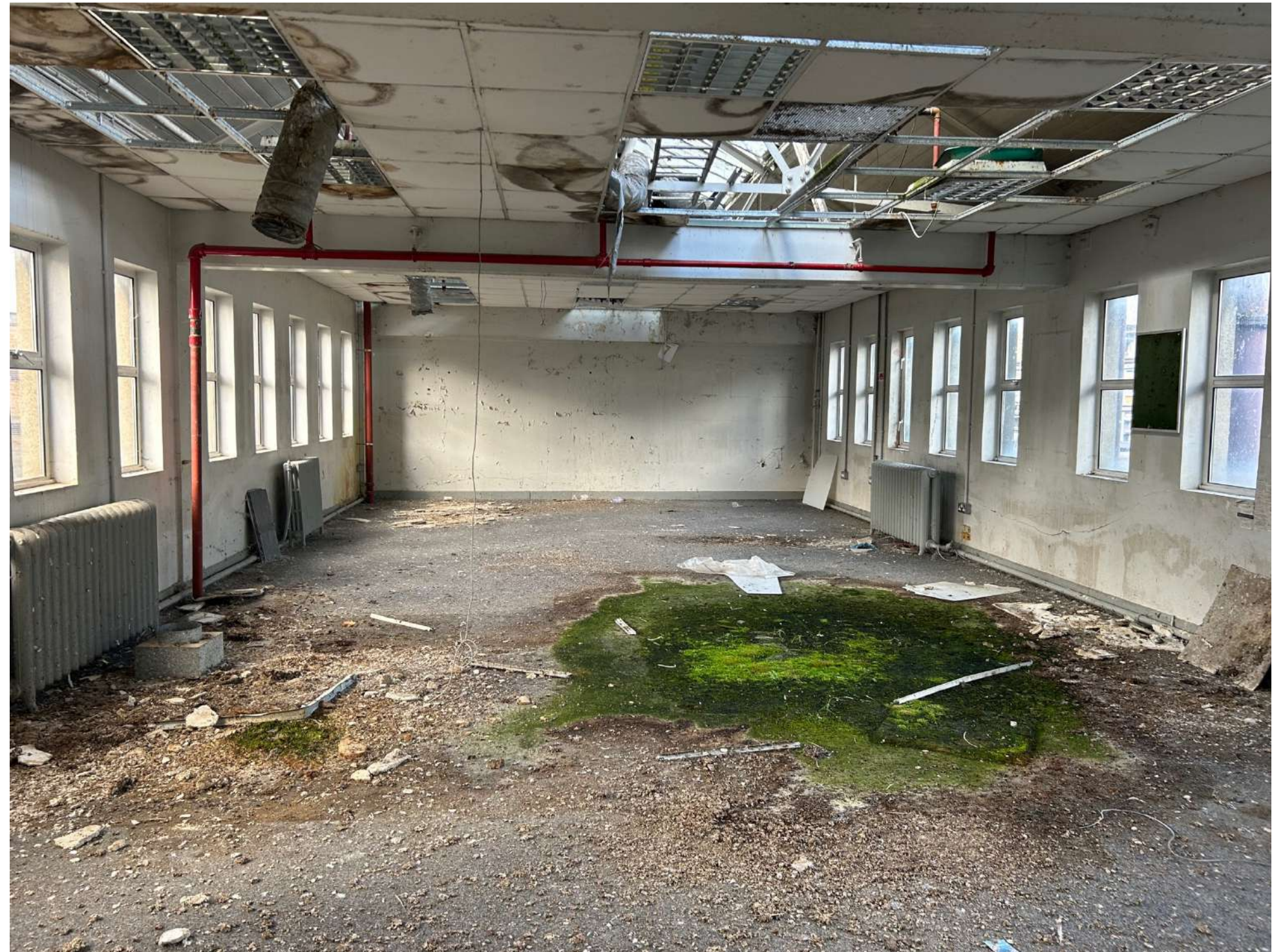
Plate 281: Top floor (former library). Steel truss pitched roof, with north facing rooflights, in poor condition, above contemporary suspended ceiling panels. Contemporary windows frame to north and south elevations. Sustained water ingress and pigeon guano has resulted in deterioration of the building fabric.
