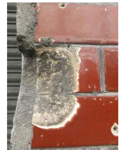
Plate 46: The former vehicular entrances are framed in a brick which red/orange glazed finish. Note impact damage. Also, the bull-nosed detail has been removed and the reveal rendered. It is intended to reinstate the original bull-nose detail using special bricks to match the existing.
