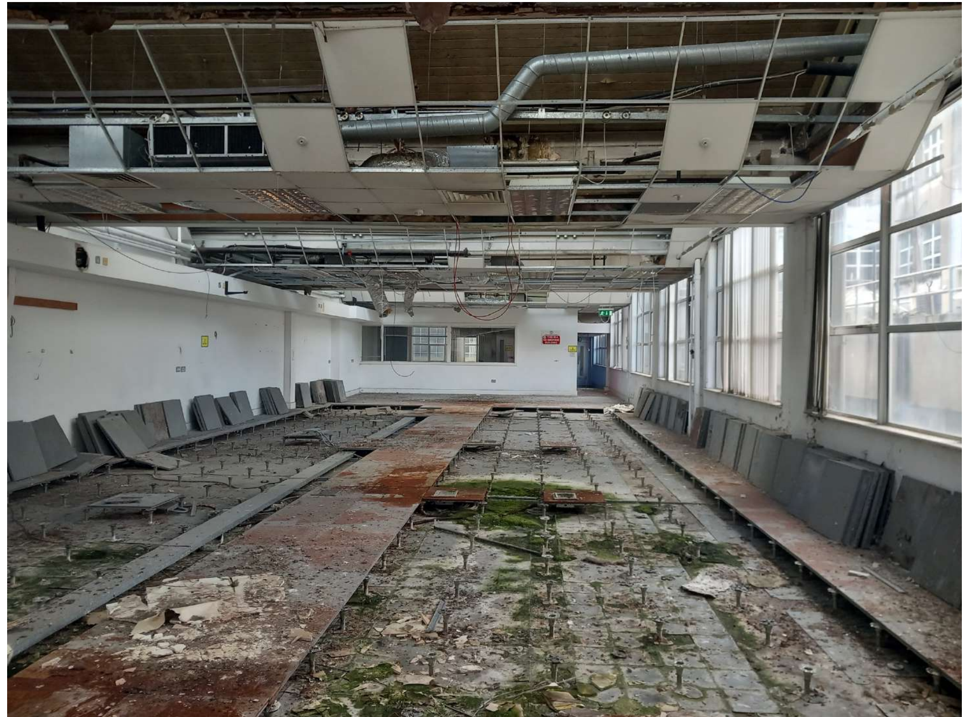
Plate 279: View facing south towards contemporary partition. Sawtooth roof above contemporary suspended ceiling. Contemporary windows. Raised access floor. Damage due to sustained water ingress.
