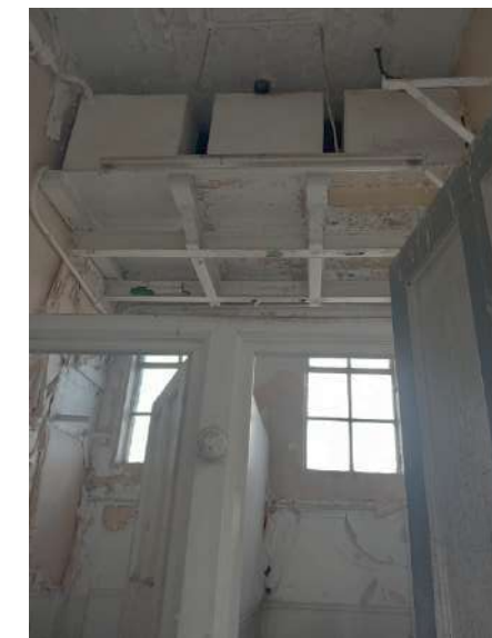
Plate 158: Water tanks supported above cubicles on the top floor level.
