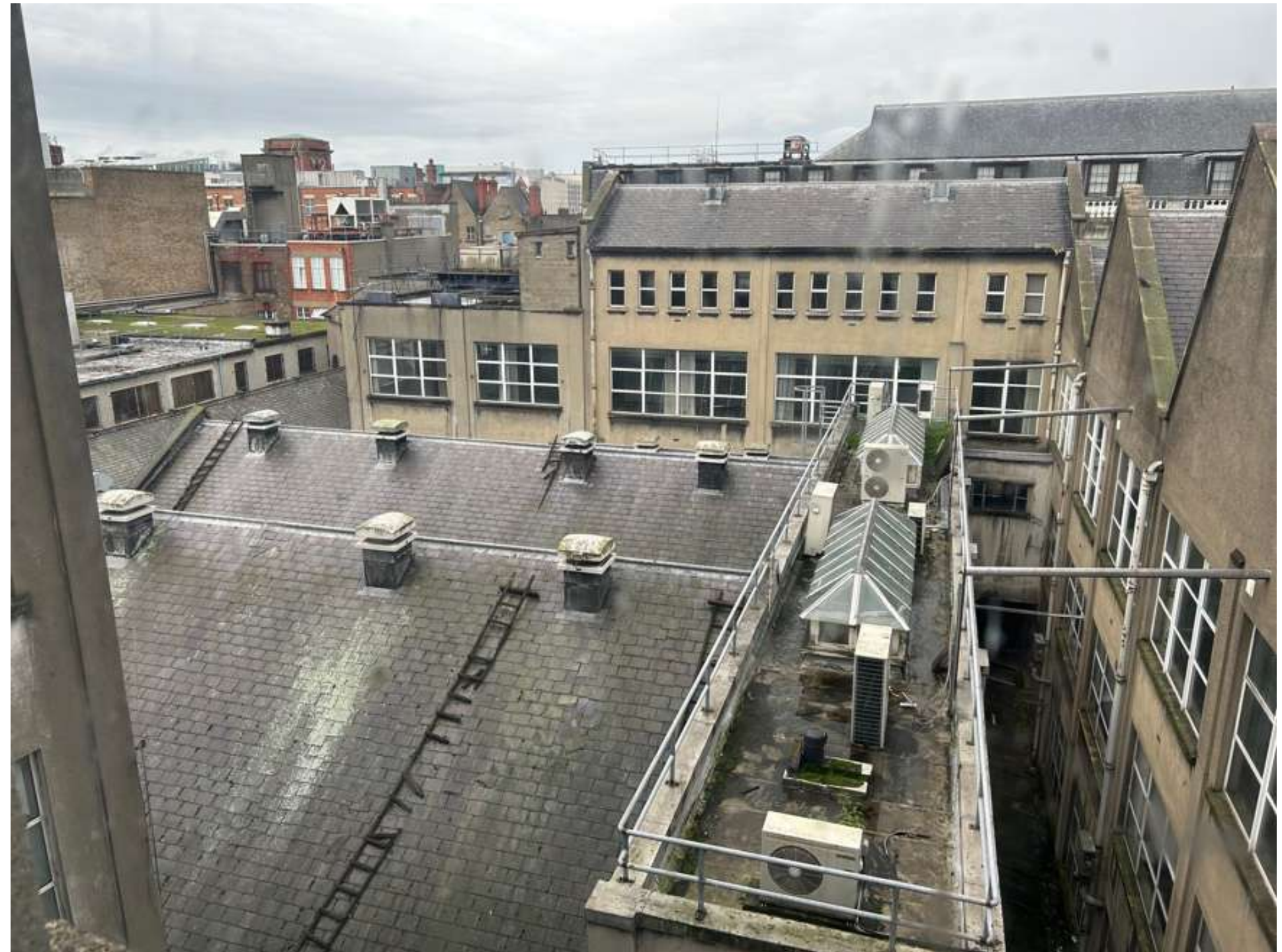
Plate 186: View over the machine room roof towards the rear (south) elevation of Area. Slate roof finish to south facing pitch, with rolled lead ridge. Multiple cracked and slipped slates visible. Ventilation stacks dressed in lead.
