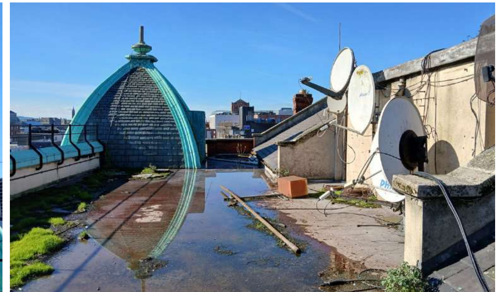
Plate 27: Main roof of Independent House facing west. The condition of the concrete roof slab has deteriorated on account of the drainage issues and degradation of roof linings.
