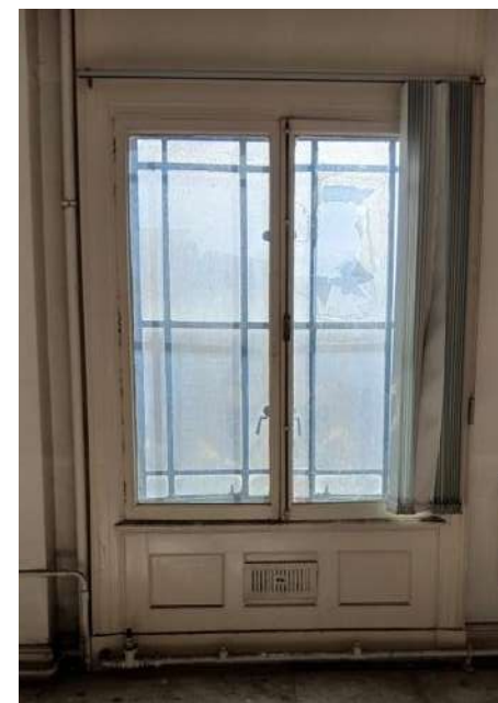
Plate 11 Typical window: the windows have timber framed secondary glazing with moulded architraves and panelled window aprons. Many of the surrounds have been damaged by the installation of pipework and services.
