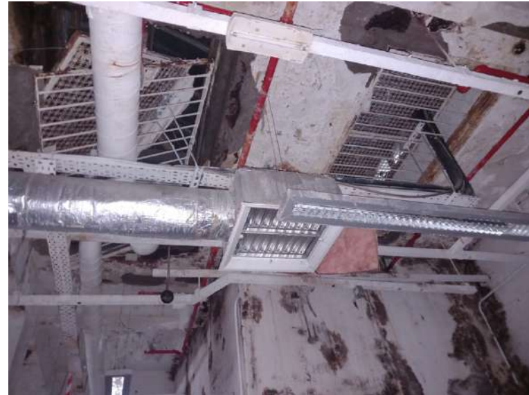
Plate 135: Concrete frame structure impacted by water ingress. Contemporary services throughout.
